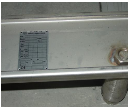
Position of the data plate : inside the cabinet B-E1 CUISPAT 1/1
