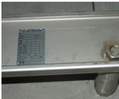
Position of the data plate : inside the cabinet B-E1 CUISPAT 1/1
